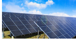
Fig.1 Photovoltaic power generation
